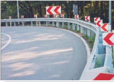
Example of a dangerous barrier (source: http://www.fema.ridersrights.org )
